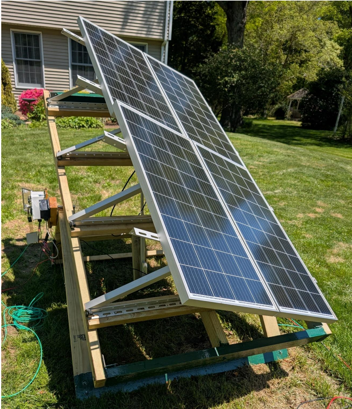
Figure 2-11. Base with Panels Mounted Outside, Left Side View. (Note: the panels are set at two slightly different elevations, showing the manual elevation increment of these racks)
